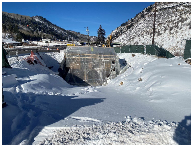
Tent over the wet well to protect and heat it during concrete curing
