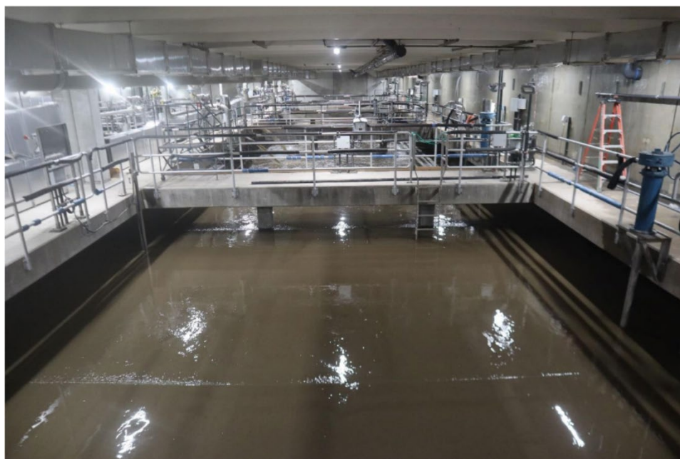
Upstream end of Aeration Basin #1 process train shortly after achieving normal operating level.
