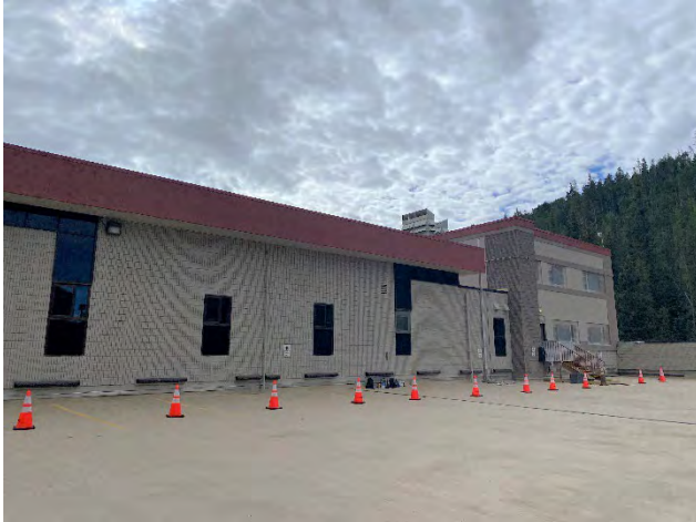
Paint on the back of the building
